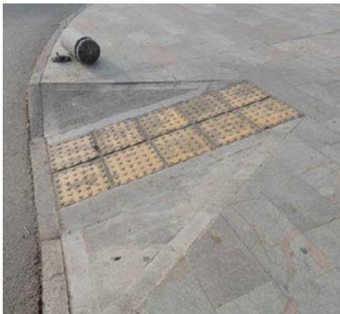
Pavement designed to ensure easy accessibility for all persons Rio Negro, Colombia © Thamara Fortes
